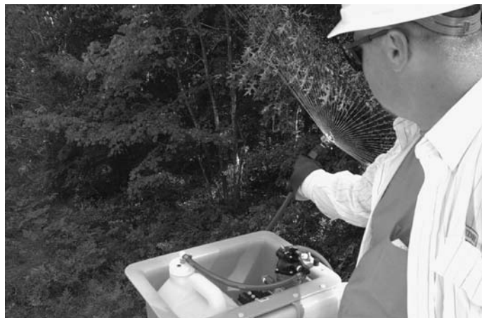
Asplundh Crew Leader John Hymer demonstrates the self-contained Thinvert Side-trimm'r™ application system, which attaches to the bucket of an aerial lift. A Widecast™ #1554 nozzle makes a 15-foot swath of uniform droplets containing 10% Krenite® S blended with 90% Thinvert RTU®.
